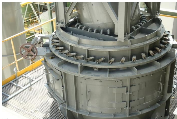
Figure2. Air separator TSV DN3200 used in closed-cycle cement grinding
