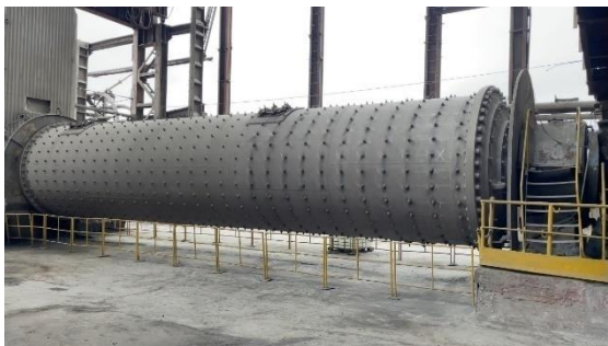
Figure 1. Cement tube mill 3,2x15 m
